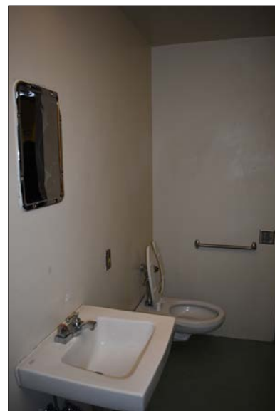
Figure 38. Photo of Wet Cell Sink and Toilet
